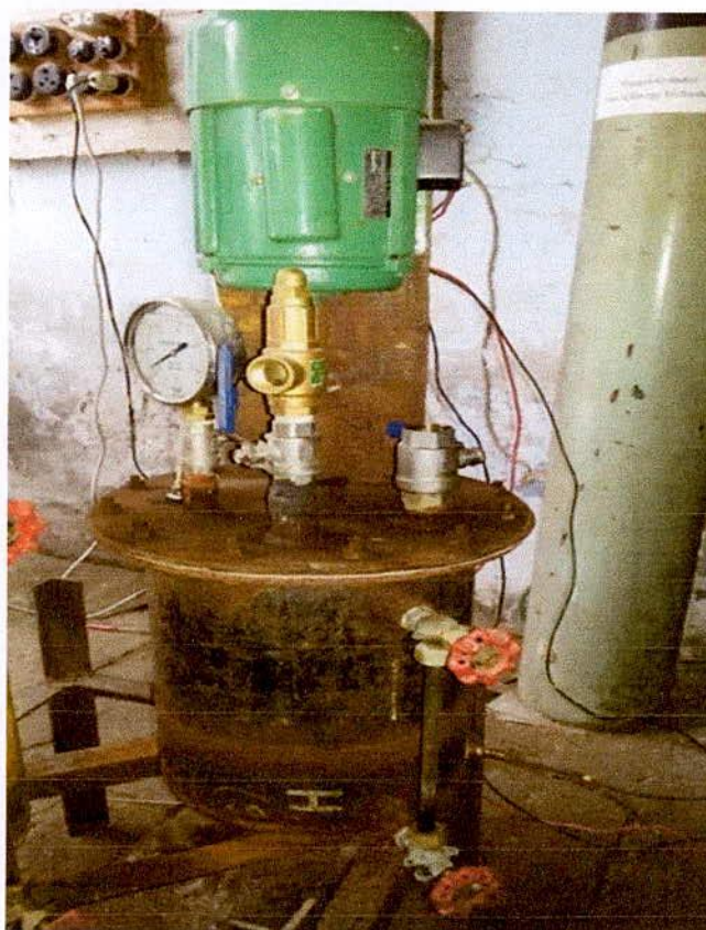
Figure 4.2: Photographic view of Reactor
