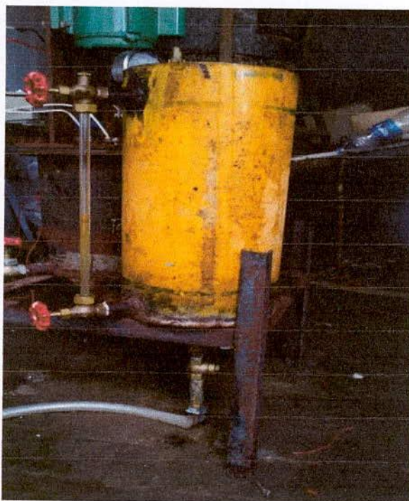
Figure 4.3: Photographic view of Washing vessel and Separator
