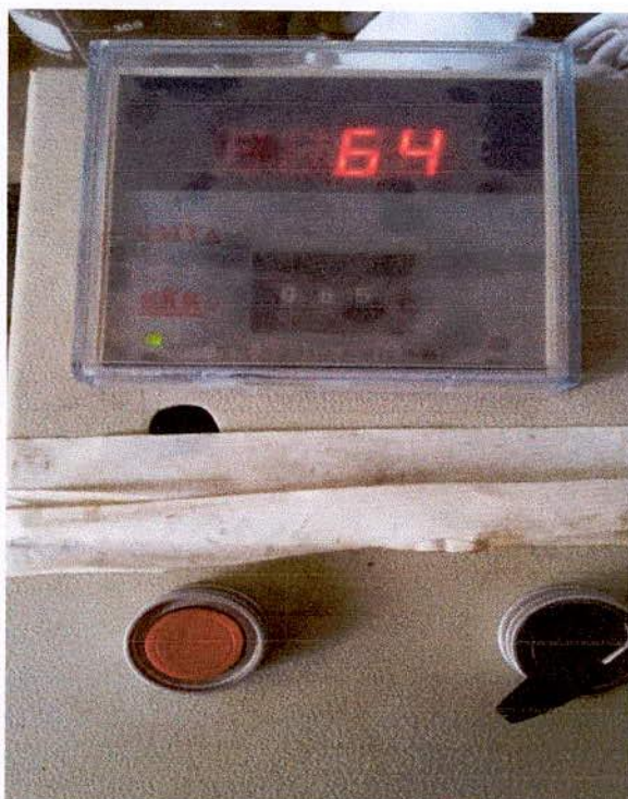
Figure 4.4: Photographic view of Temperature controller
