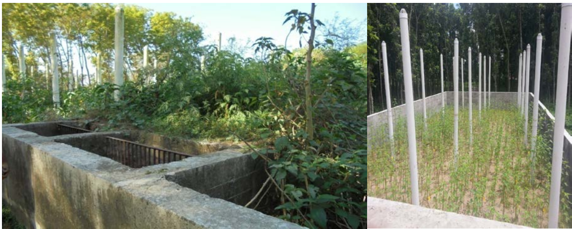
Figure 4.36: Existing Treatment Plant of Jhenaidah Municipality
