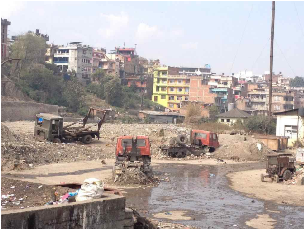
Figure 2.5: A failed Faecal Sludge Management facility in Nepal. Photo credit: ENPHO
