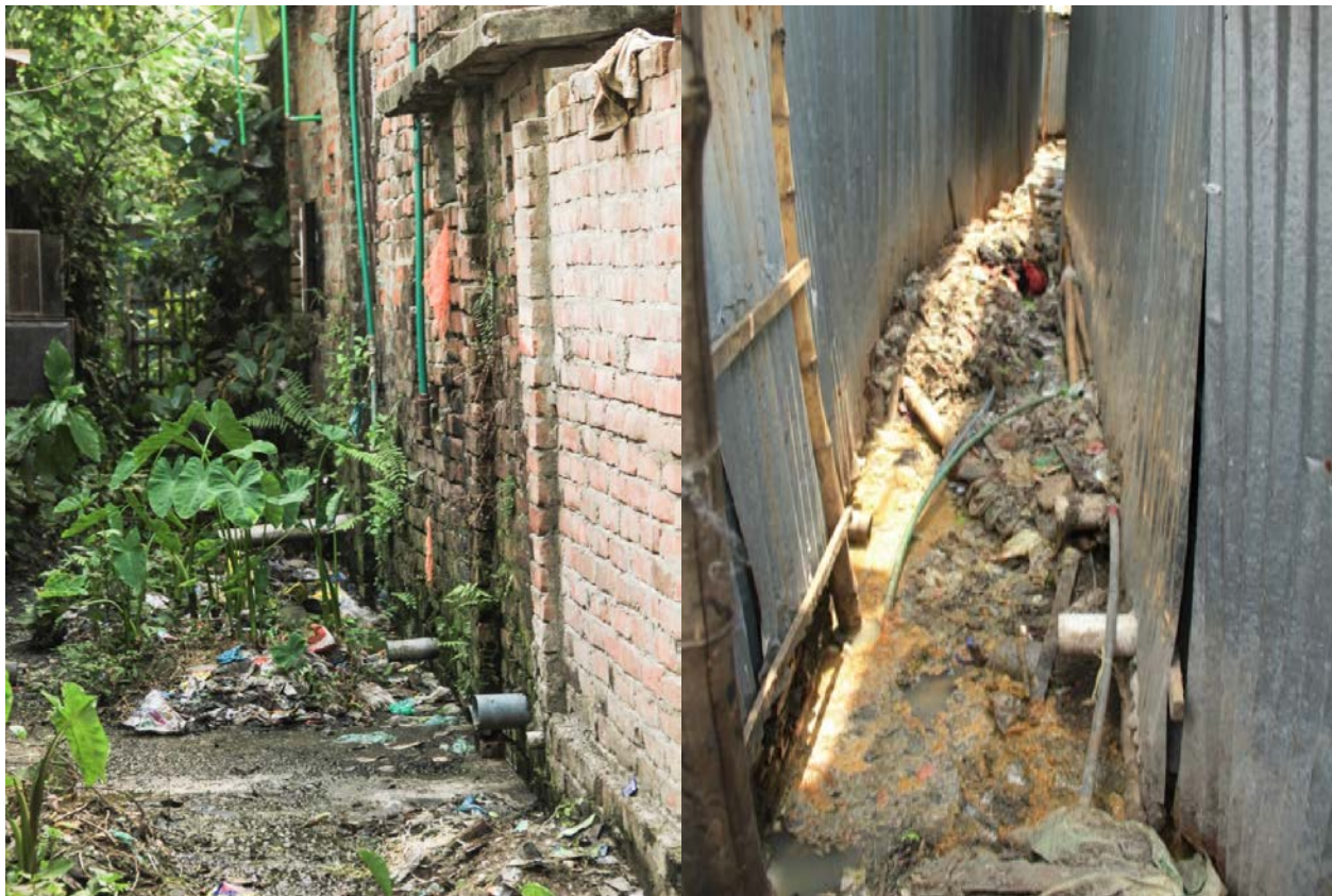
Figure 4.6: Septic tank connected to open ground
