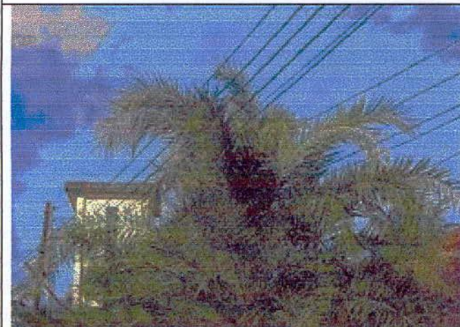
Picture-11: Line with improper clearance
