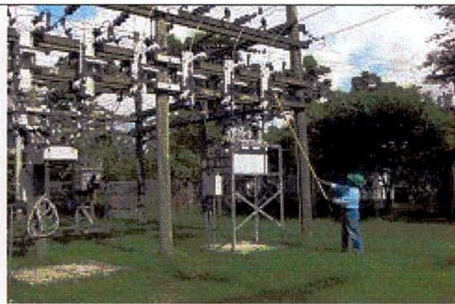
Picture-6: Line is operating a substation with proper safety
