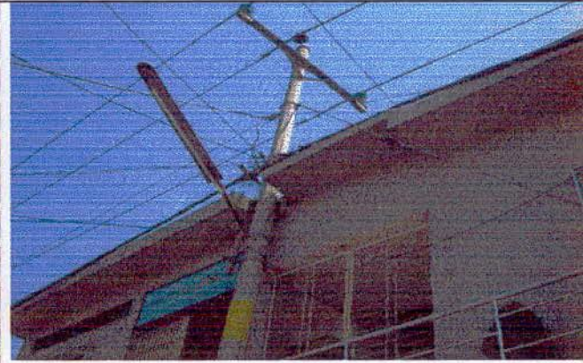
Picture-16: Line with improper clearance
