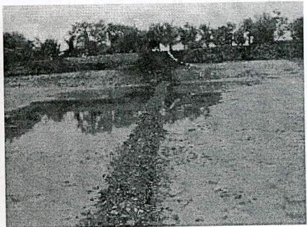
Figure 4.12 Leachate collection pipe with brick aggregates as filter media
