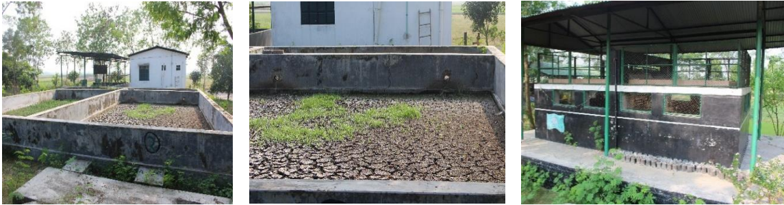
Figure 4.5: Existing Treatment Facilities of Kushtia FSTP (Drying Bed, Cocoa Pit Filter)
