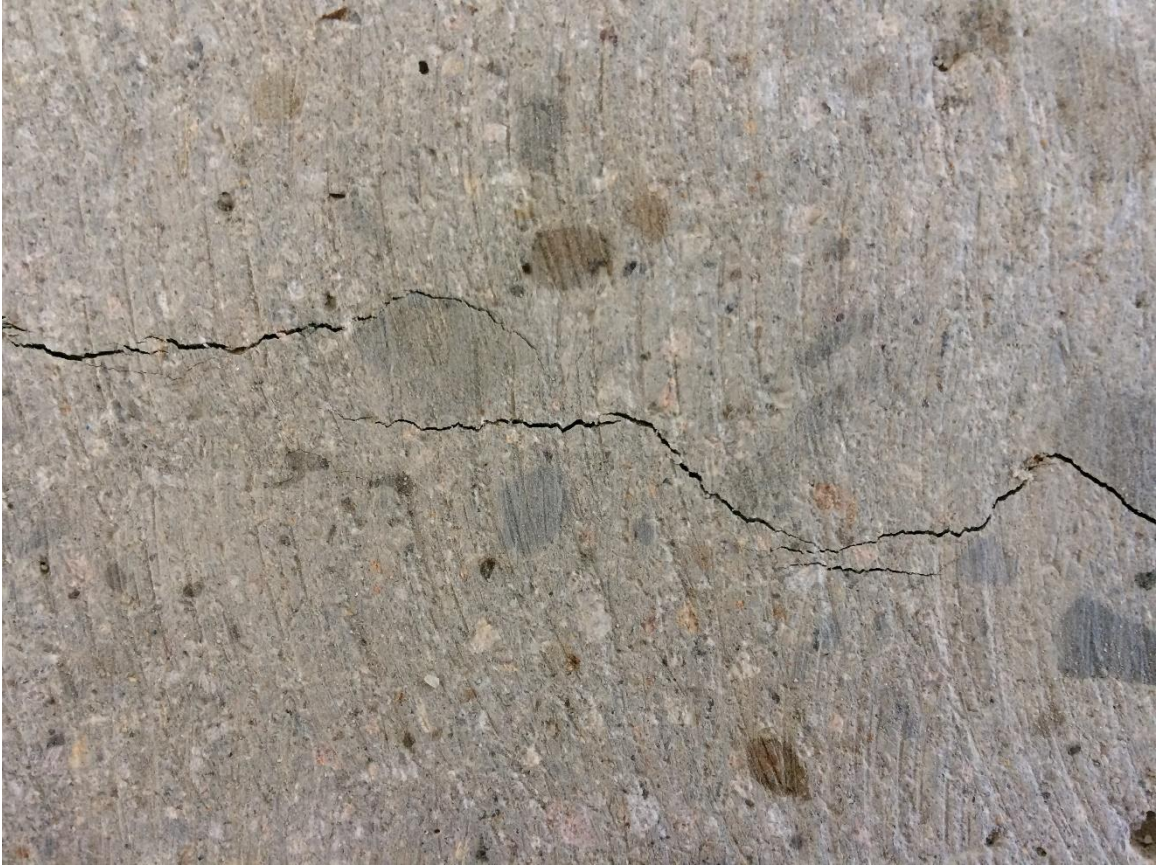
Figure 4.18: Longitudinal Crack Pattern of Beam VII (C = 50 mm)
