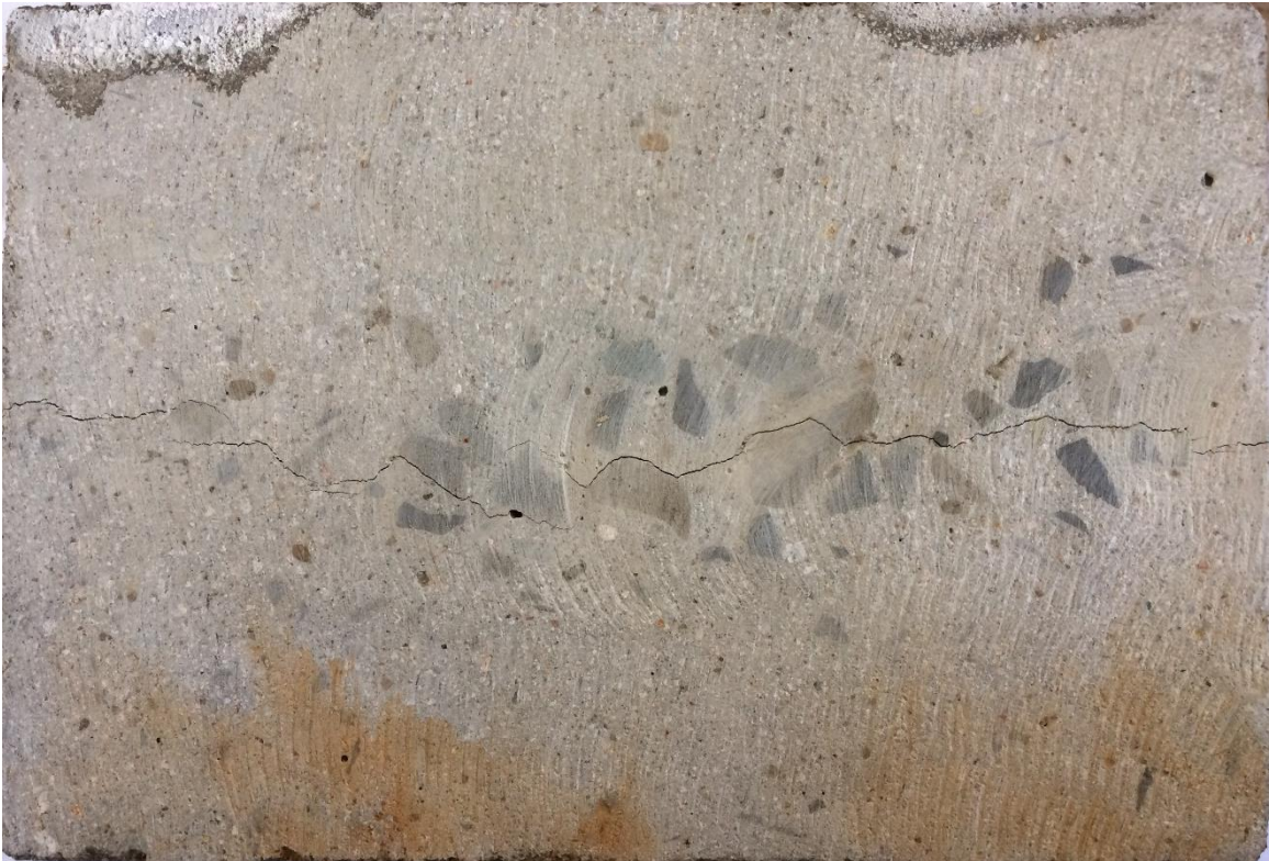
Figure 4.17: Longitudinal Crack Pattern of Beam V (C = 37.5 mm)
