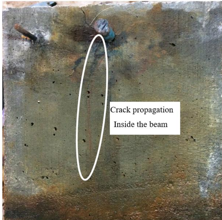
Figure A5: Propagation of Cracks inside the Beam ( C = 20 mm)
