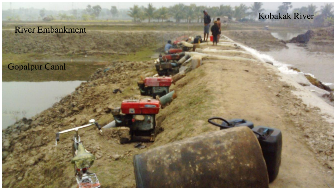
Figure 5.32: Pumping of stagnant water to the river Kobadak of the study area
