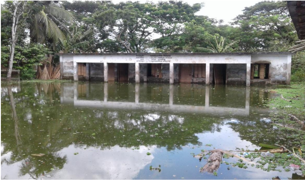
Figure 5.11: Prolonged water logging in the primary school in the study area
