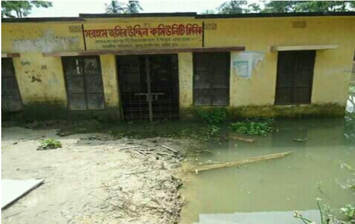
Figure 5.10: Affected community clinic by prolonged water logging in the study area
