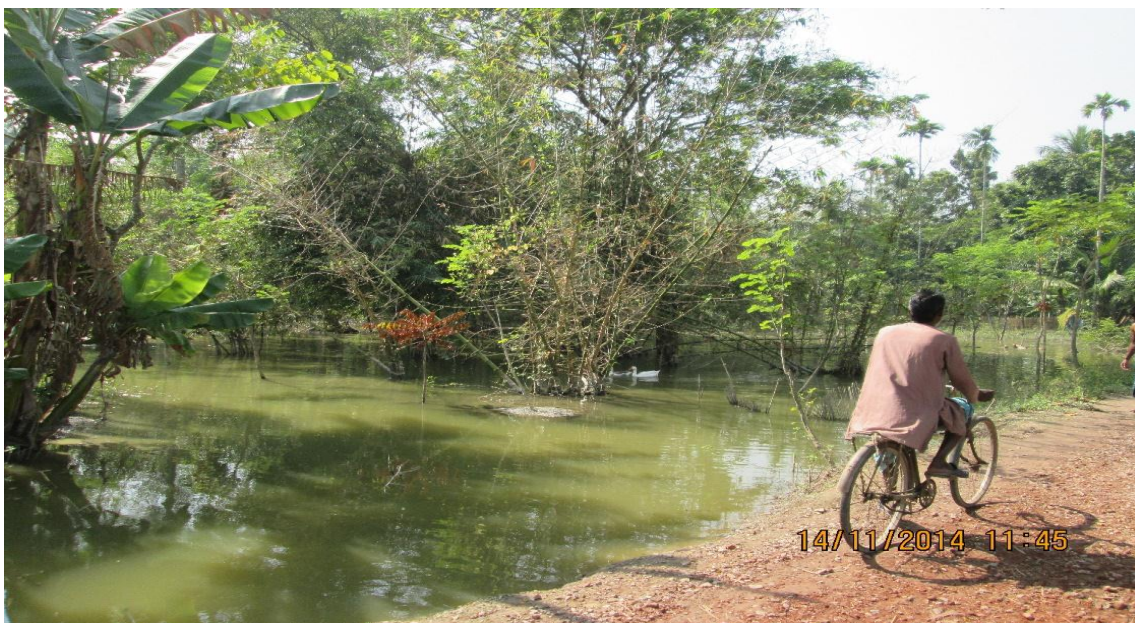
Figure 5.8: Pukka road damaged due to water logging in the study area
