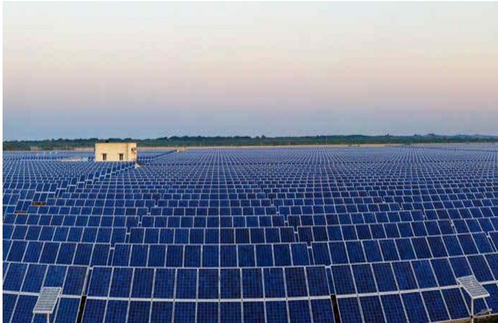
Fig: 2.6: 17 MW Mithapur solar power plant, Gujarat in January 2012 (India) [37].
